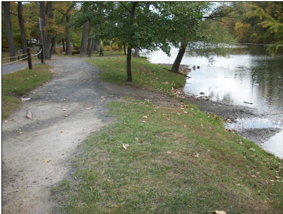
Site Photo 8: Outlet area from parking lot catch basin (erosion and sediment deposition evident)
