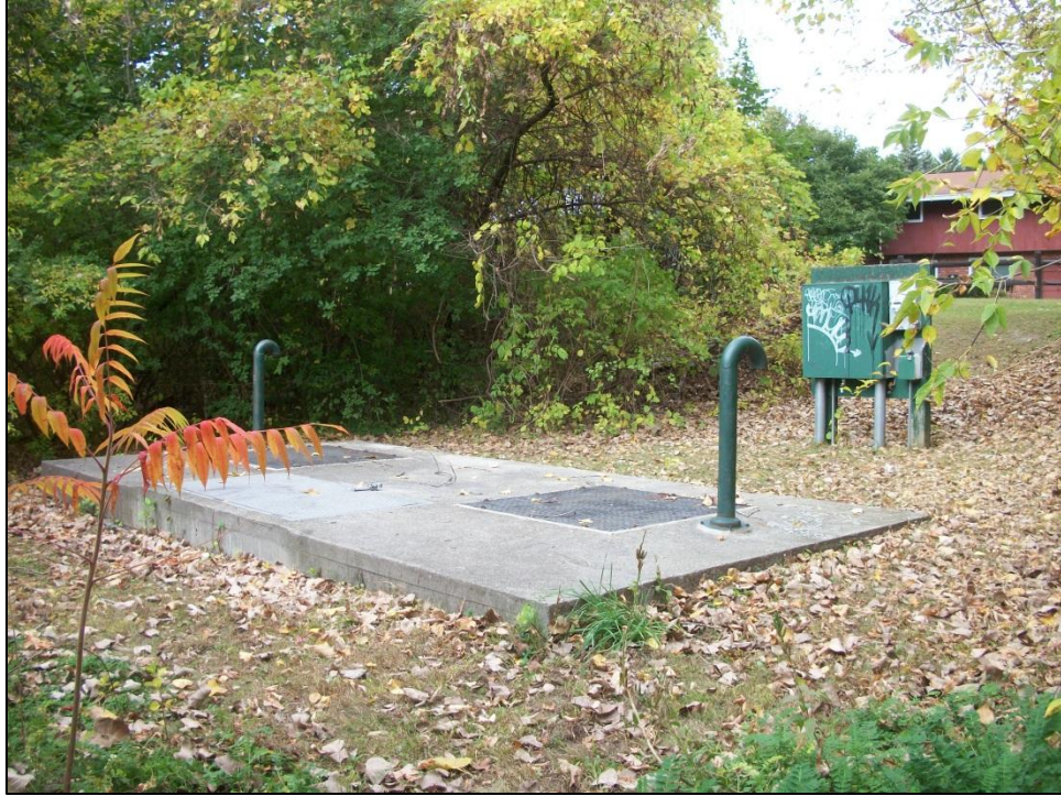
Site Photo 13: Pump Station
