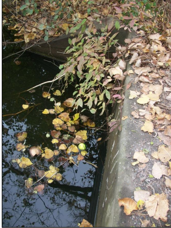
Site Photo 1: Equalization pipe between stilling basin and pond
