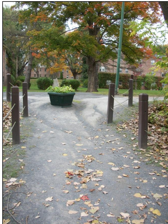
Site Photo 10: Erosion west (downgradient) of trench drain
