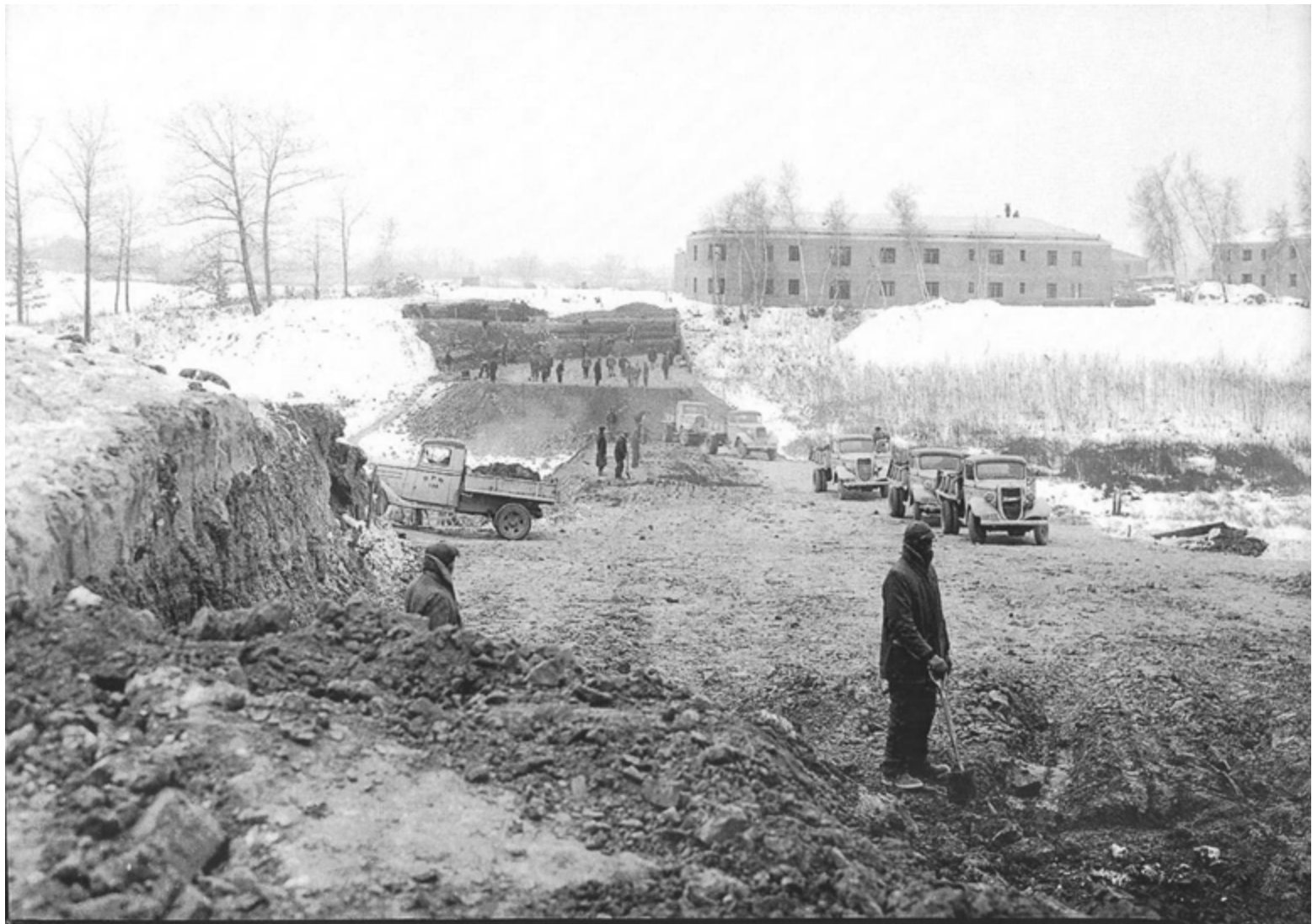
Photo showing Colonial Avenue under construction in 1941 Note Stonehenge Gardens under construction
